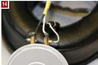
Completed connector wiring
